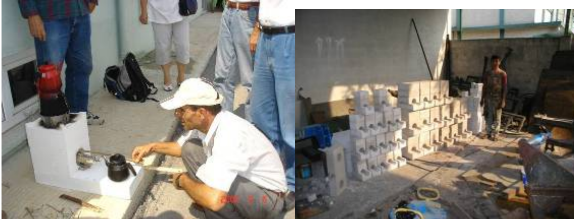
These Ytong rocket stoves are based on Larry's Ten Rules of Combustion.
